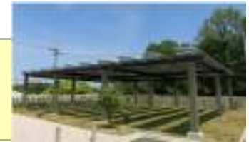
Solar power generation system (17.1 kW) above a regulation reservoir (in the communal space)
