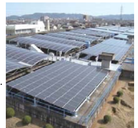
〈The solar power generation system installed at the Tsuru-Shinden water treatment plant (Kigyoyokyu (Bureau of Business Affairs) of Okayama Prefecture)〉
