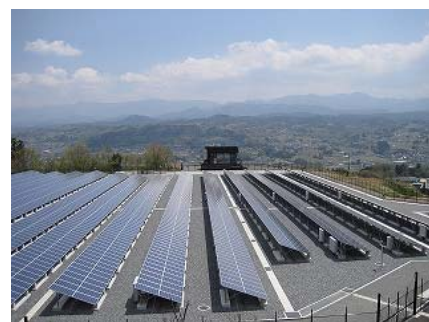
Mega Solar Iida
