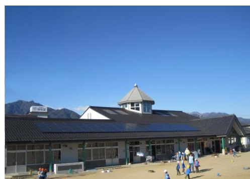
Solar panels installed by citizens fund: Kanae Mitsubo Nursery School
