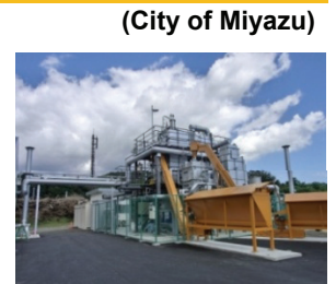
〈Biomethanol production and power generation facility〉
