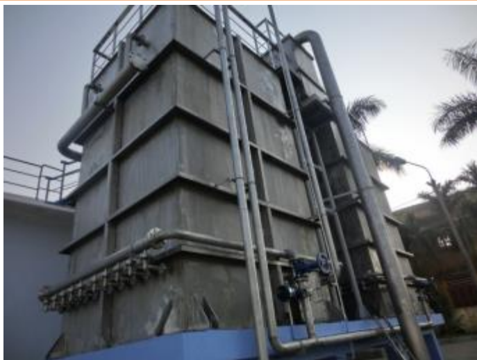
U-BCF plant in operation in Haiphong, Vietnam
