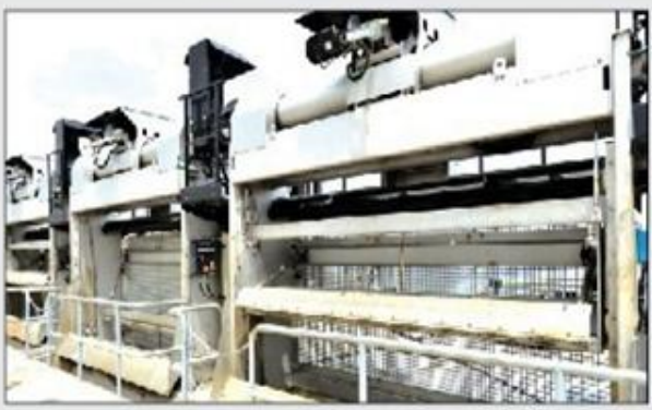
Seawater enters the plant and passes through filter screens and auto strainers.
