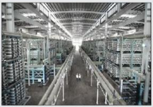
After ultrafiltration, the water goes through a two-stage reverse osmosis treatment process to remove salt.
